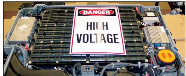
Figure 65: High-voltage battery and cooling system. Source: NAFTC.
