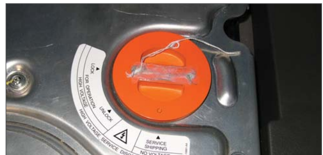
Figure 68: Hybrid high-voltage system disconnect. Source: NAFTC.
