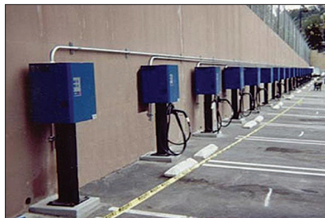
Figure 12: Level 2 Minit-Charger private fleet charging infrastructure. Source: Minit-Charger.
