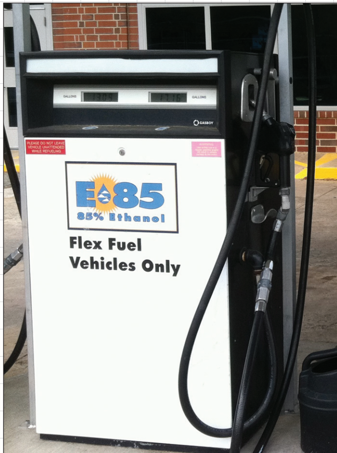
E85 pump at the UNC fuel station. Photo courtesy of UNC.
