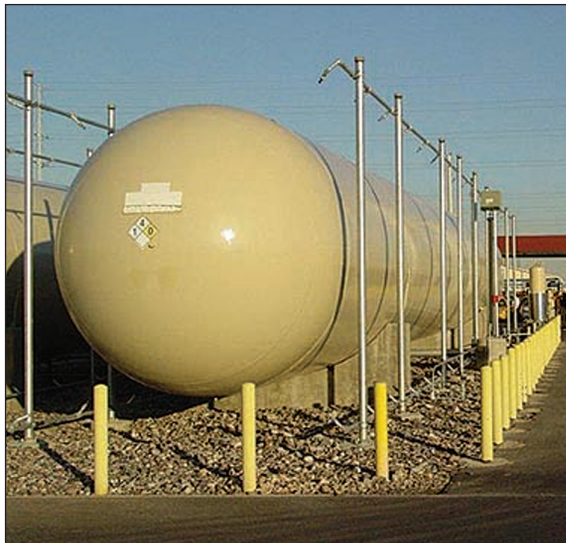
Figure 6: Large LPG storage tank for propane vehicle fueling station. Source: NAFTC.
