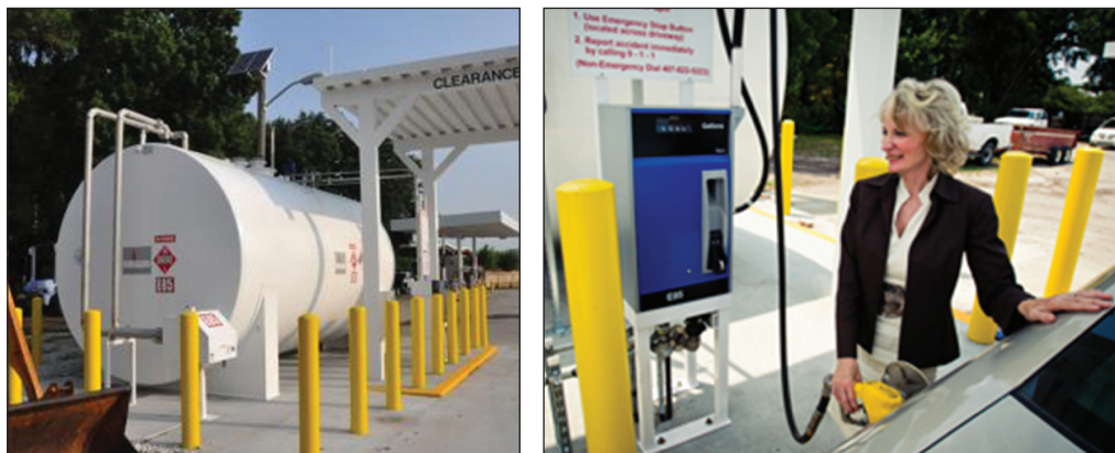
Figure 15: University of Central Florida's E85 onsite fueling station and fueling infrastructure. Source: University of Central Florida.
