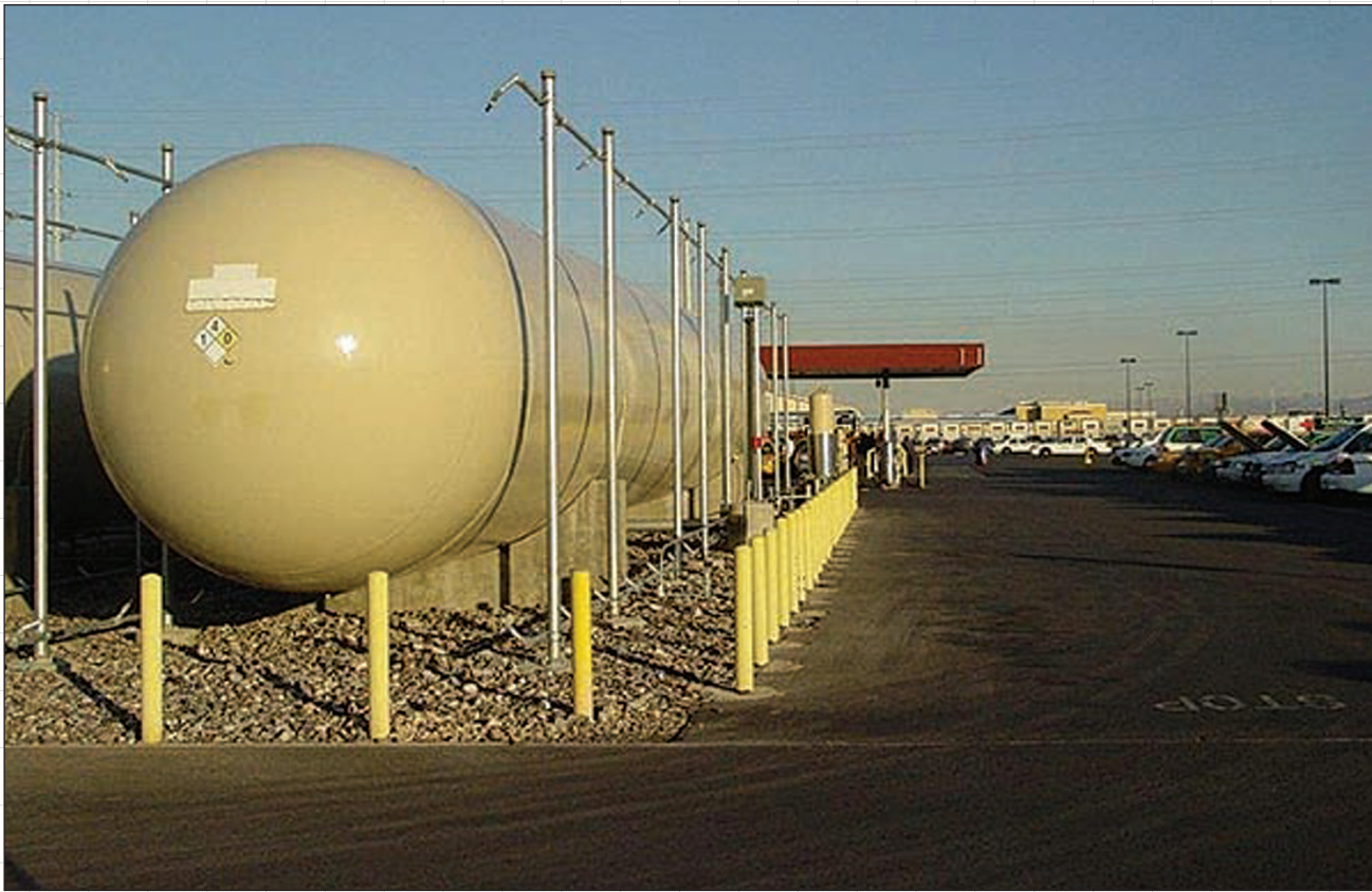
YCS propane storage tanks in the foreground are located adjacent to the fueling station seen in the background. Photo courtesy of YCS Transportation.
